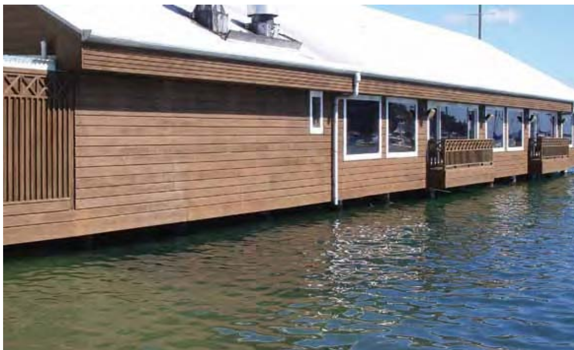
46: SYDNEY HARBOUR, DOUBLE BAY Limited clearance to the floor of the sailing club premises. Photo: Craig Morrison, Sydney Coastal Councils Group.
